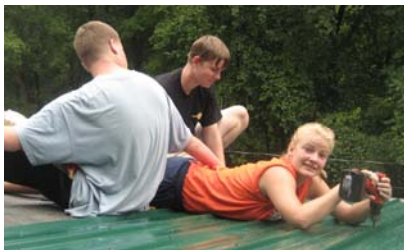
Ian Leaird, Bryan Foster and Rosalee Townsley put their roofing skills to work.
